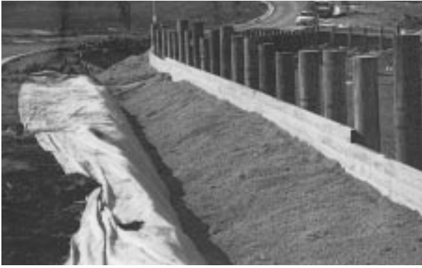
Western Earth Moving chose FBA from Vales Point to provide a drainage layer for a subdivision at Parklea.
