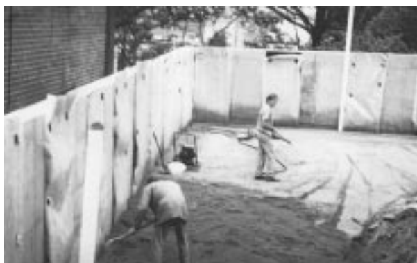
The same ash was chosen by Newcastle Pavements as a sub-base 2 to 3 m thick under a car park for a block of flats constructed by Active Developments.
